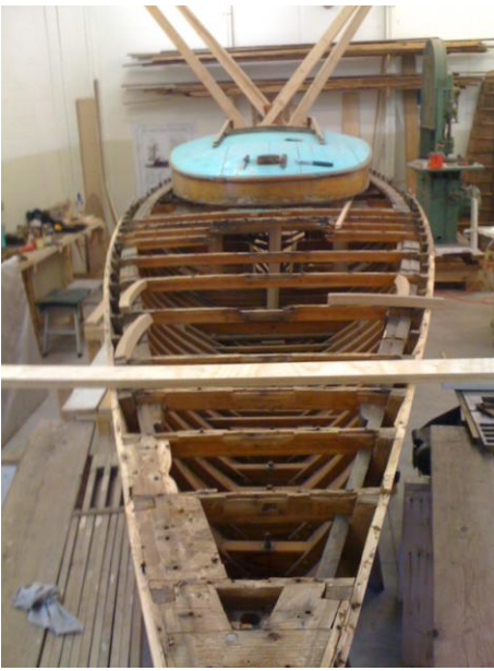
The 1958 Bill Livingston-built Witchcraft , getting new deck beams, deck, sister frames, etc. Stop by on Tuesday nights and lend a hand.
